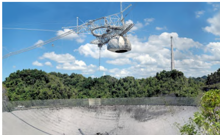
The vertical "boom" pointing down into the dish is the 96 foot long antenna that fell.
